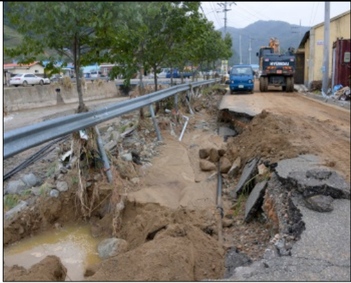
Damaged road (Yeongdeok)
